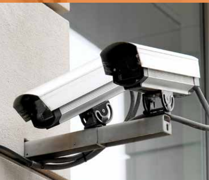
SECURITY: PERIMETER CAMERAS, 24/7 PATROLLING, ACCESS CONTROL AND VISITOR VERIFICATION
