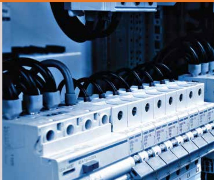
CONNECTED POWER LOAD OF 7-14 KVA DEPENDING ON TYPE OF APARTMENT
